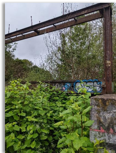
Figure 2: Charterhouse Sluice gate, blocked by Japanese Knotweed, covered in graffiti. 2021
